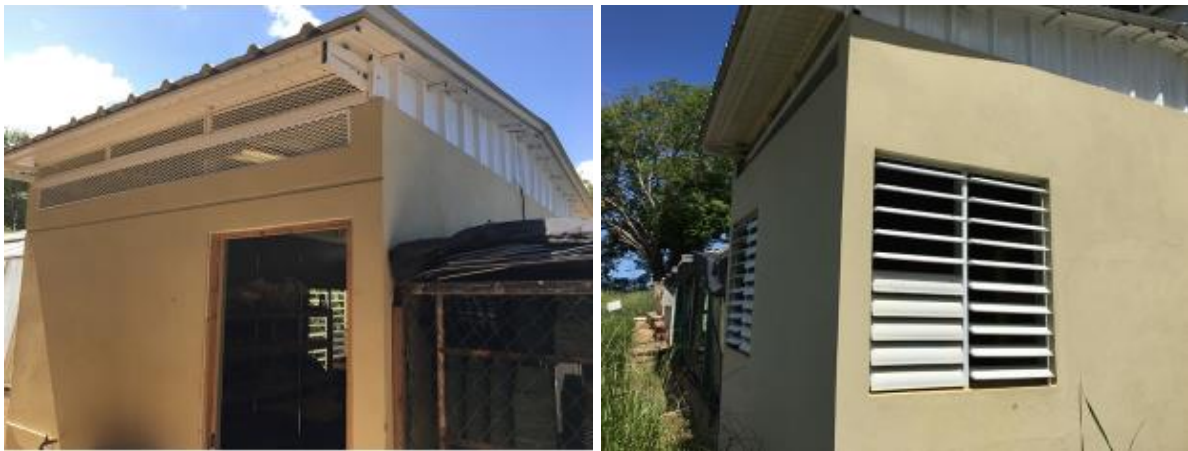
P027/27A/27B Storage is a 3-compartment storage area constructed of reinforced concrete for the roof, walls and floor. Each compartment has a door
