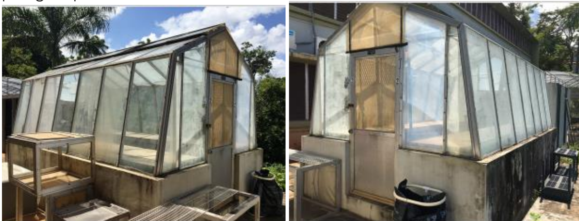
P024 Agricultural Greenhouse is a greenhouse that is constructed of metal framing situated on a concrete slab with a 3-foot concrete wall. The exterior consists of 2x6 plexiglass panels.
